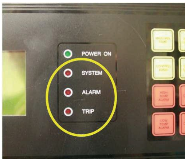
Figure 10: Common System, Alarm, and Trip LEDs
